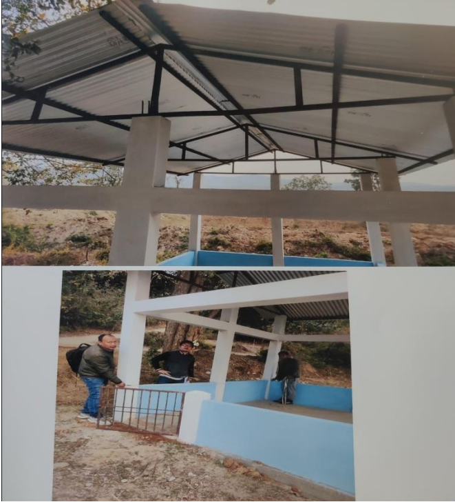
Name of work:-Construction of social centre 2 at Khejurbond Name of Scheme:-Axom Adarxo Gram Yojana
