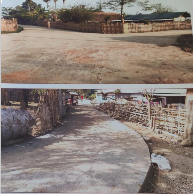
NAME OF WORK: - CONSTRUCTION OF CEMENT CONCRETE PAVEMENT AT PRASADIMDIK NAME OF SCHEME: - AXOM ADARXO GRAM YOJANA 2019-20.
